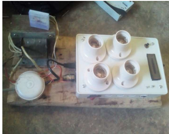
Figure 9: Implemented Transformer Overload Protection System
