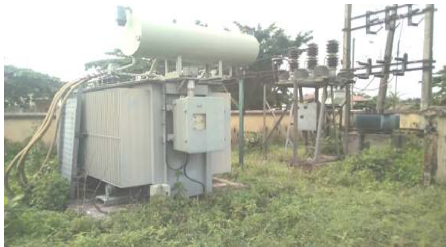
Fig.2. DELSUTH 7.5MVA, 33/11 injection Substation.
