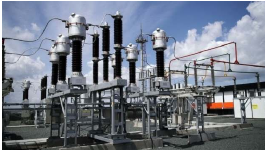
Figure 2: A Transmission Station in Abuja
