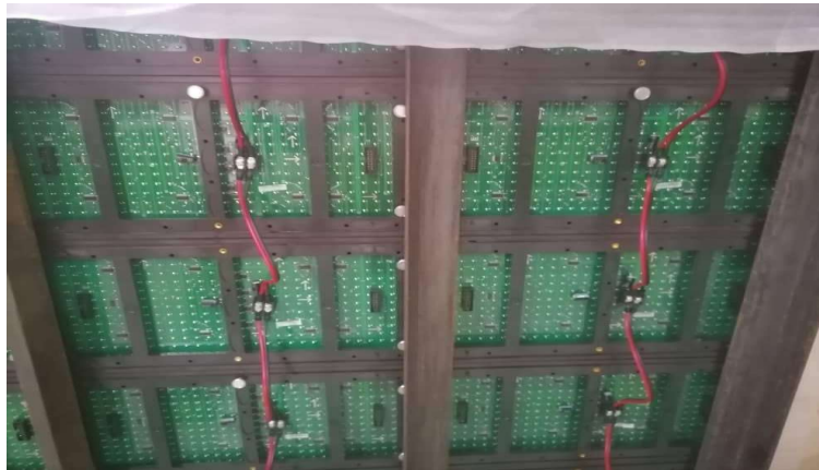
Figure 16: Cables Arranged in Parallel from One Board to Another
