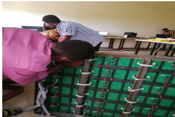
Figure 15: Cables Being Arranged in Series from one Board to Another Board
