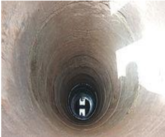
Figure 2: View into a hand-dug well cased with concrete rings
