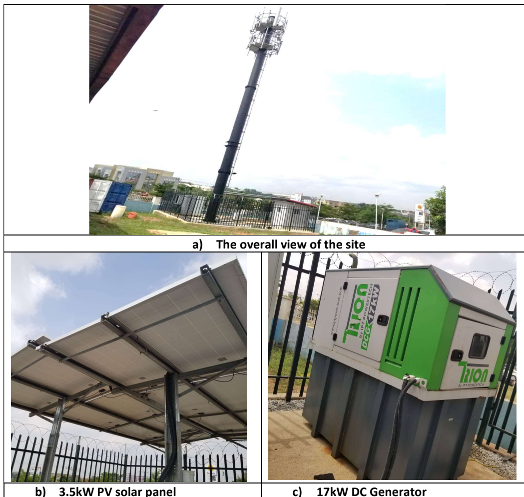
Fig.1: Mabushi telecommunication substation, Abuja Nigeria
