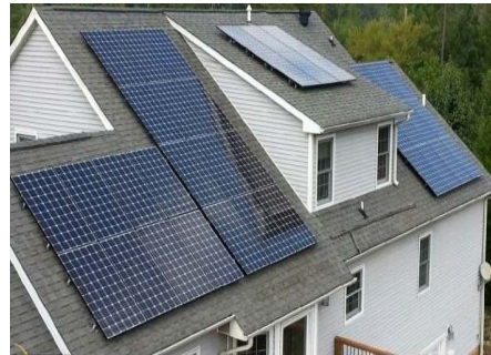
Figure 4: Roof mounted PV Solar Array
